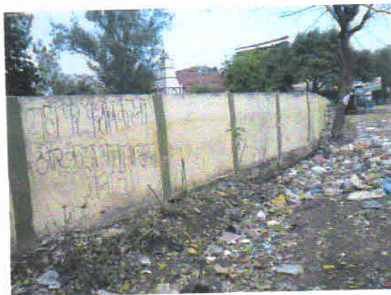
PICTURE 5.2: DISPOSAL OF SOLID WASTE IN STORM WATER DRAIN
