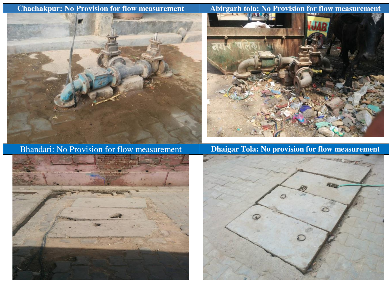
Figure 20 Photographs Captured at Submersible Pumping Stations
